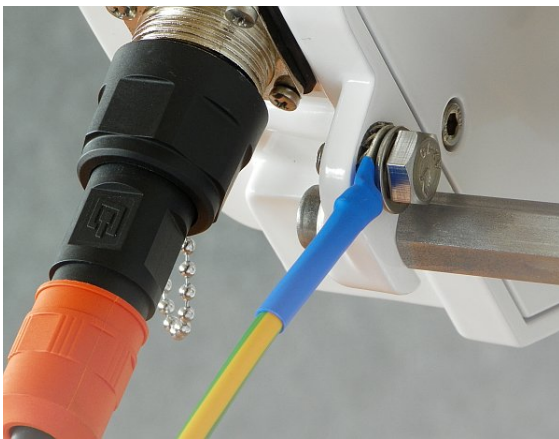
Fig. 5.67: Protective conductor at the FOD unit
