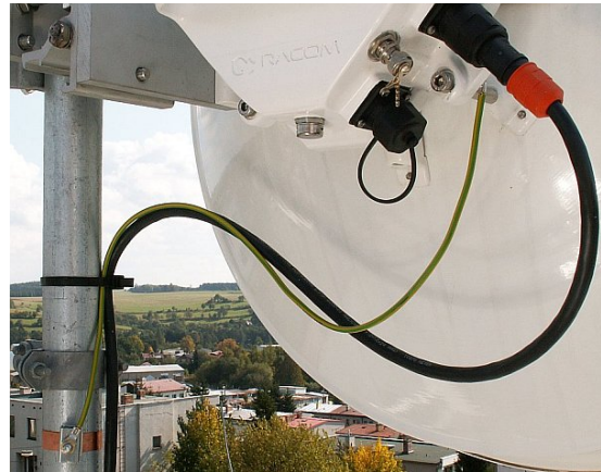
Fig. 5.66: Grounding the FOD unit
